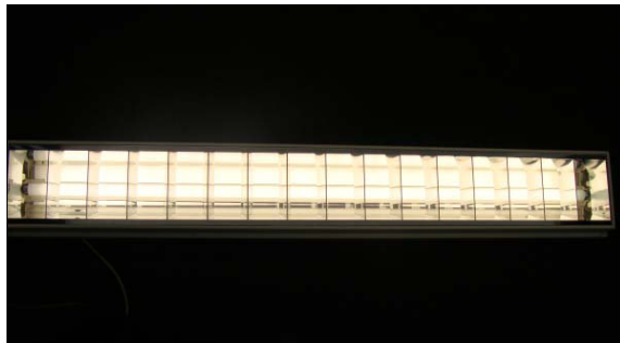
Figure 9.22: Luminaire # 3 switched on.
