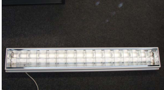
Figure 9.21: Luminaire # 3 switched off.
