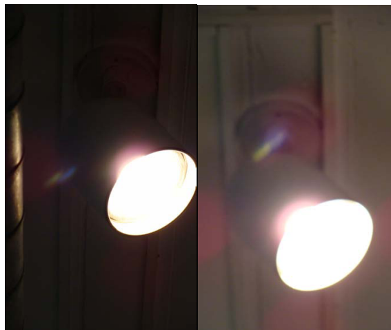
Figure 9.40: Two photos of luminaire # 6 switched on.
